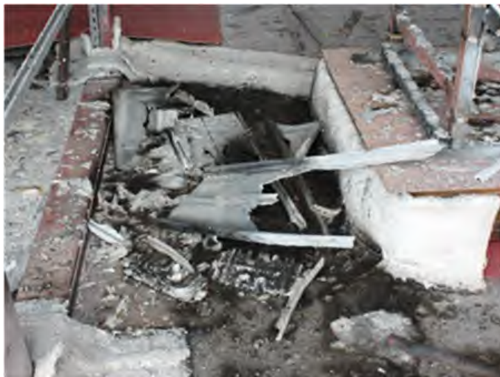
Fig. 208. Post-Experiment 2-41 Bus Duct. Remaining bus duct enclosure located on ground after experiment.
