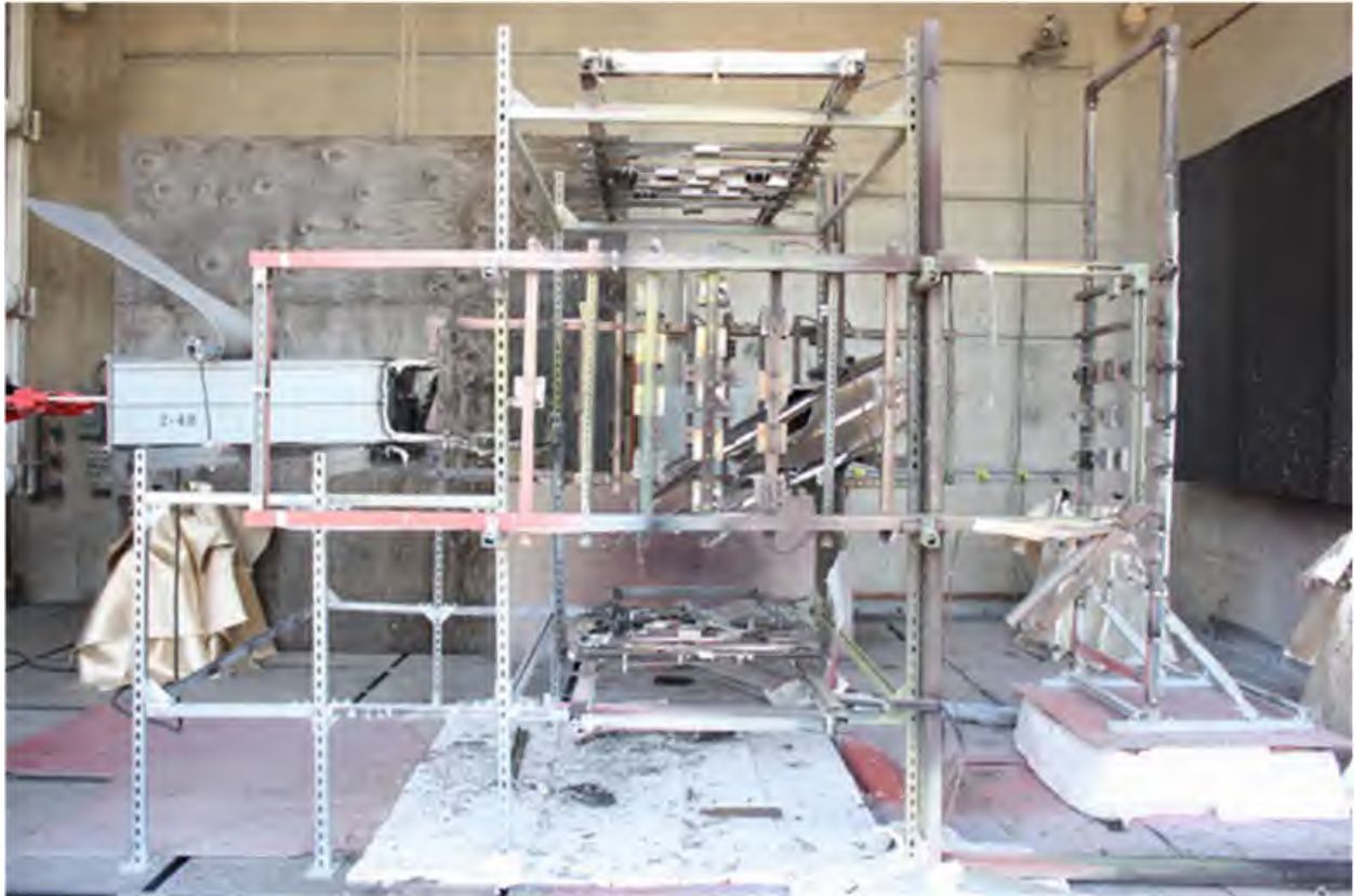
Fig. 202. Post-Experiment 2-40 Bus Duct. Duct severed with a portion resting on the support structure.
