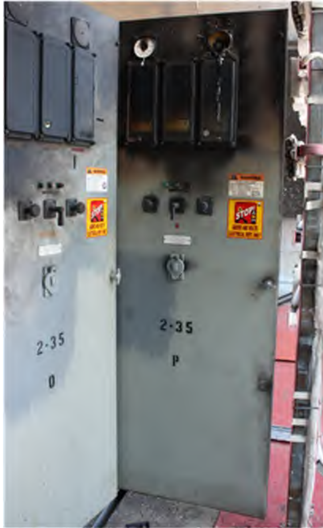
Fig. 180. Post-Experiment 2-35 Enclosures “O” and “P”. Soot and heat damage on front enclosure doors.
