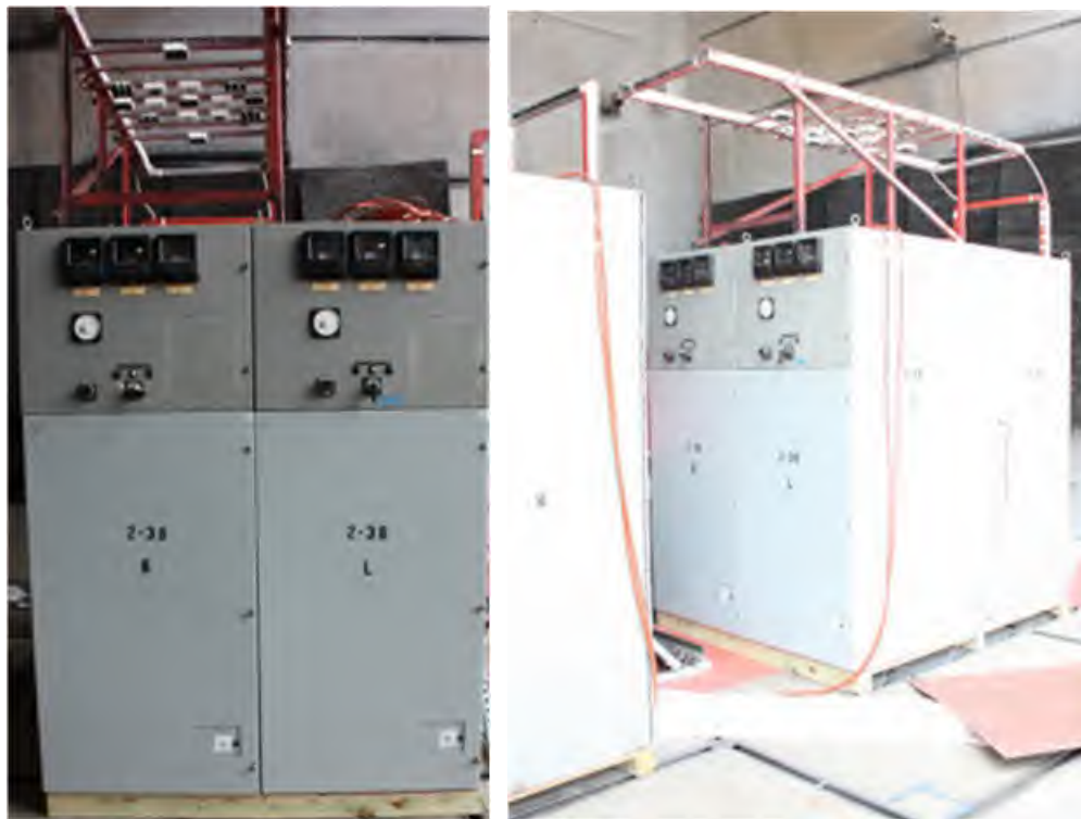
Fig. 190. Pre-Experiment 2-38 Enclosure “K” and “L”. Left – Enclosure “K” (left) and “L” (right). Right – general cross-aisle configuration with Enclosure “M” across from “L” and Enclosure “I” across from “K”.
