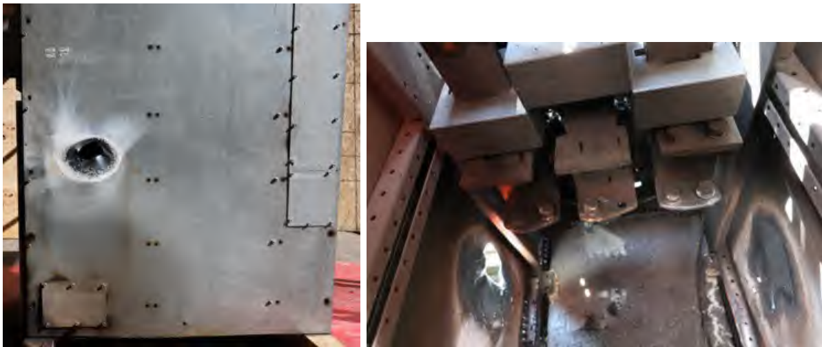
Fig. 215. Post-Experiment 2-XXA. Left – enclosure breach on right side of gear (cladding 1.5 mm [0.060 in] thick), Right – internal bus bar condition at arcing location.
