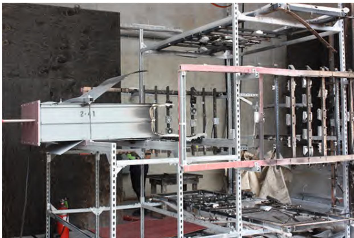
Fig. 206. Post-Experiment 2-41 Bus Duct. View of remaining duct from power side.
