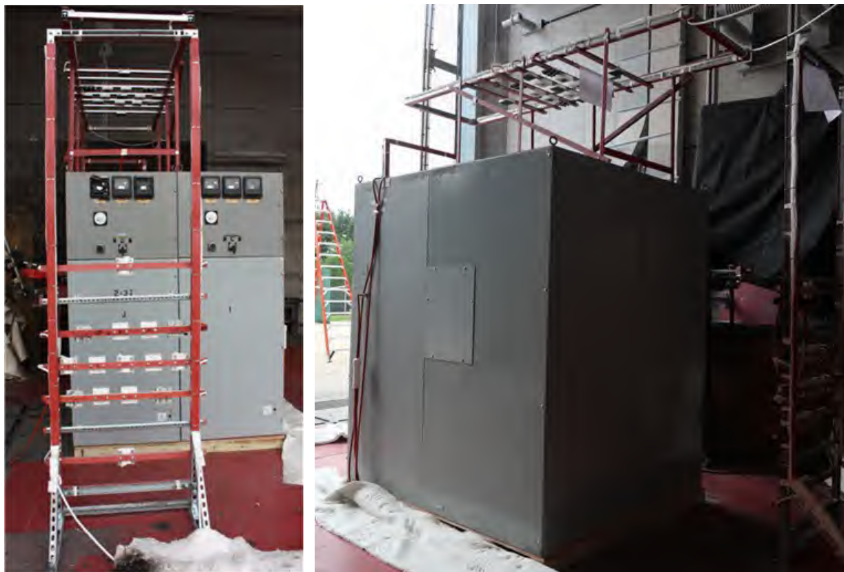
Fig. 59. Pre-experimental setup for experiment 2-37. Left – Front of switchgear showing Enclosure "J" left where arc was initiated on breaker stabs and Enclosure "I" to the right, Right– rear angle view showing general experimental configuration with Enclosure "I" to the left.
