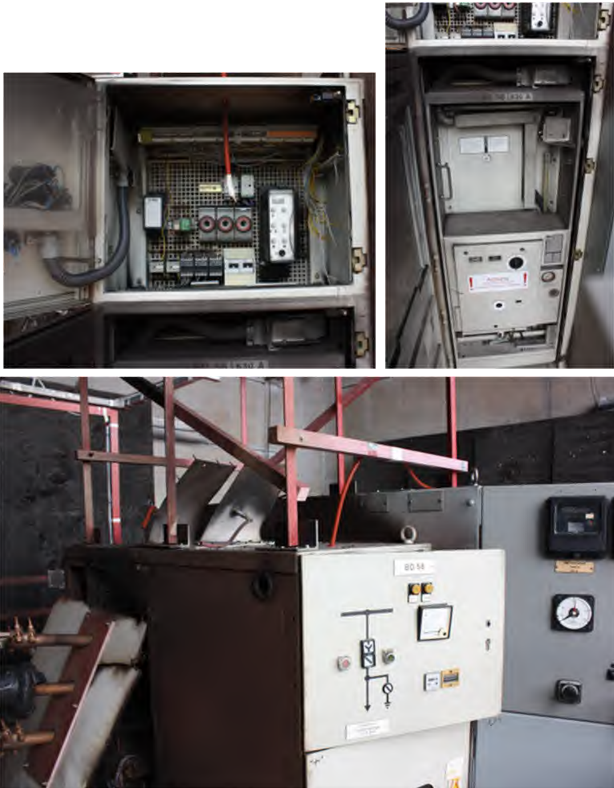
Fig. 183. Post-Experiment 2-36, Enclosure "H". Top-left – front instrument cubicle, Top-right – lower breaker cubicle, Bottom – exterior showing two panels re-oriented on top of enclosure, one panel on side completely disconnected from enclosure.
