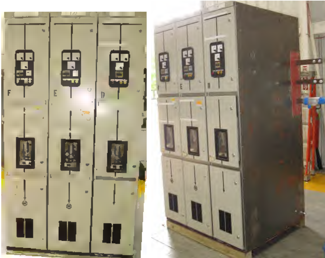
Fig. 17. Photographs of the low-voltage lineup configuration.
