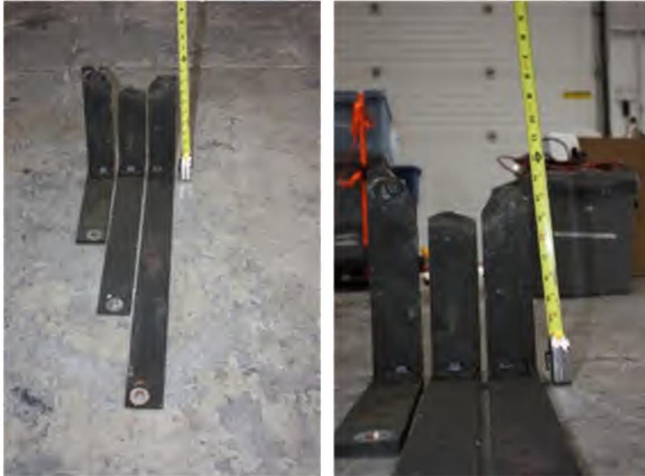
Fig. 38. Photos of Experiment 2-33B vertical supply bus bars post-experiment. Location with material loss (top of image) is where the bus connected to the breaker. Bar orientation as shown in photo is C-B-A.
