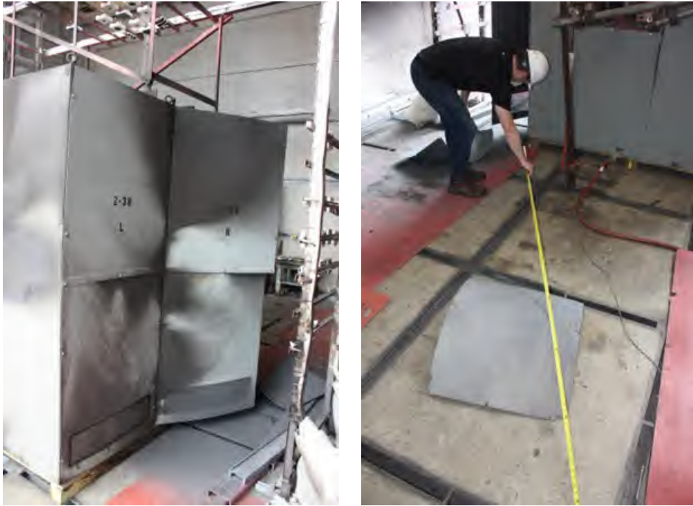
Fig. 193. Post-experiment 2-38 Enclosures “L” and “K”. Left - Enclosure "K" rear panel breach due to pressure, Right – measurement of rear internal panel distance from Enclosure “K” corner. Note that both internal panels surrounding main bus were ejected during experiment and located on floor. Farthest panel was approximately 3 m (10 ft) from enclosure, while nearest panel was approximately 0.9 m (3 ft) from enclosure.
