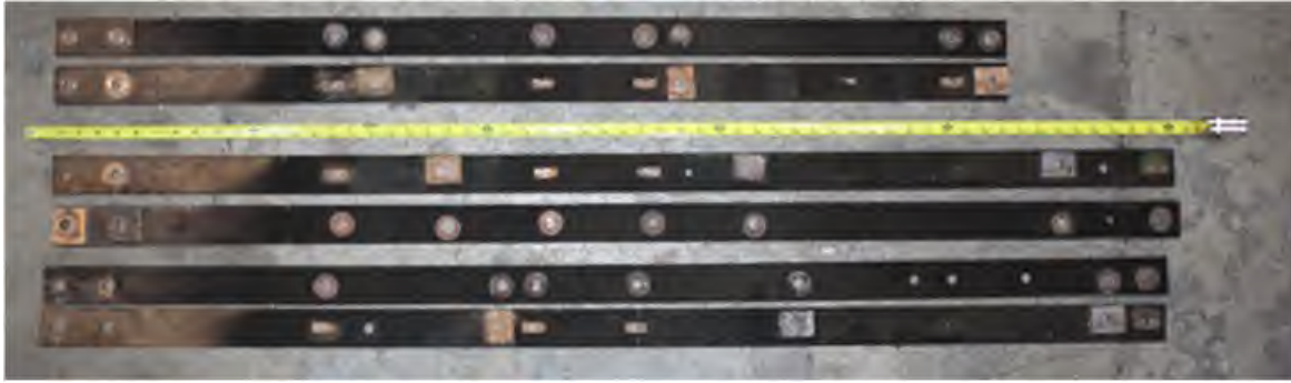
Fig. 172. Post-Experiment 2-33B Horizontal Main Bus Conductors.
