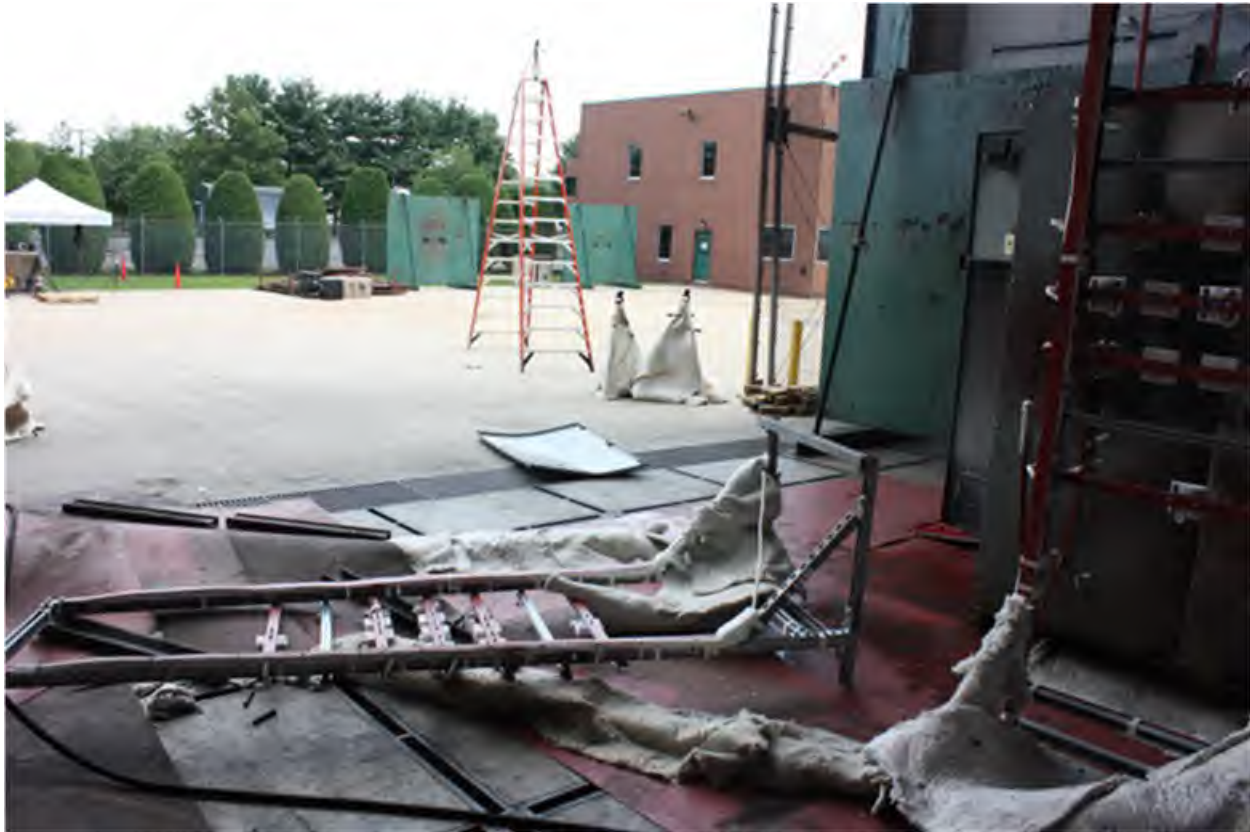
Fig. 75. Enclosure Post-Experiment 2-39. The front door is approximately 4.9 m (16 ft) from Enclosure "M". Instrument Rack #1 is laying on ground due to impact from Enclosure "M" front door during experiment.
