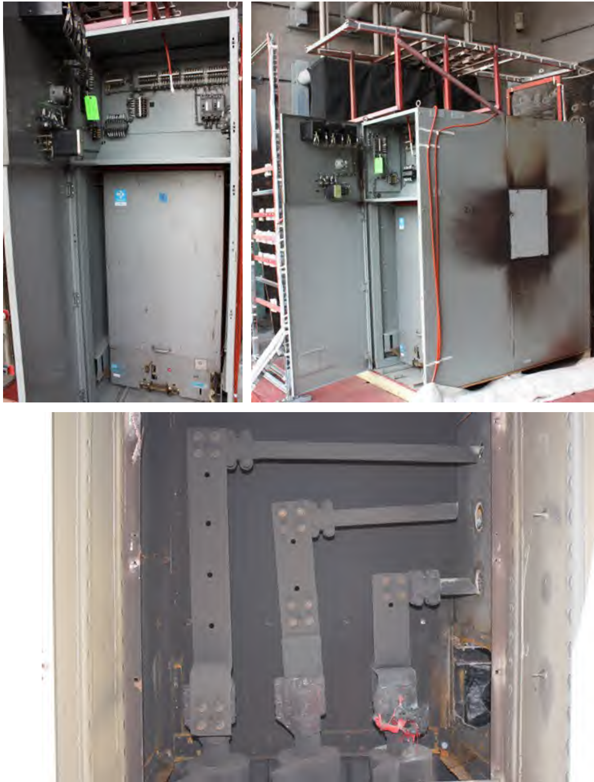
Fig. 184. Post-Experiment Enclosure "N". Top-left – front instrumentation and breaker cubicle, Top-right – side showing soot deposit near cover over main bus section of switchgear, Bottom – main bus section showing damage to horizontal copper bus.
