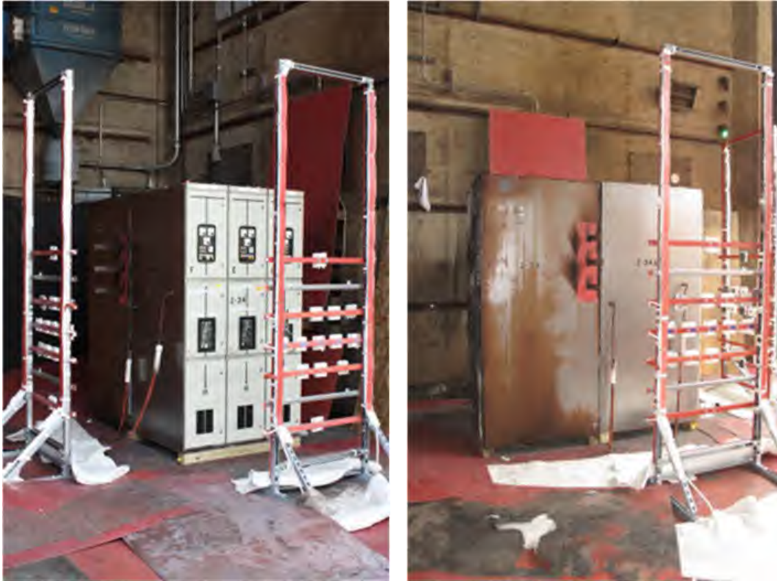
Fig. 174. Pre-Experiment 2-34 Enclosures “D”, “E”, and “F”. Left – front angle view of experimental device, Right – side view of “back-to-back” experimental configuration (note enclosure labeled 2-33 on left is not energized).
