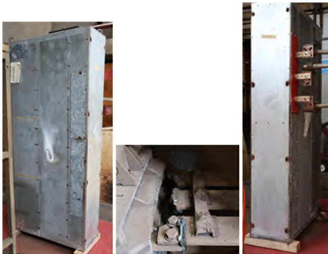
Fig. 221. Post-Experiment 2-YYA. Left – Enclosure heat damage on right side (opposite incoming power supply), Center – bus bars at arc initiation location, Right – Enclosure heat damage on left side (incoming power supply side).
