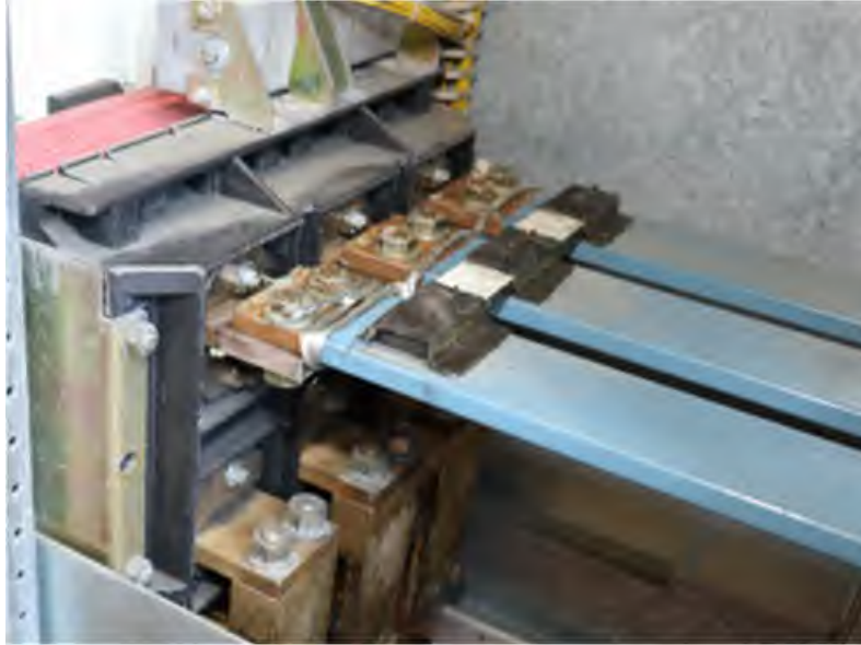
Fig. 219. Pre-Experiment 2-YYA arcing wire location.
