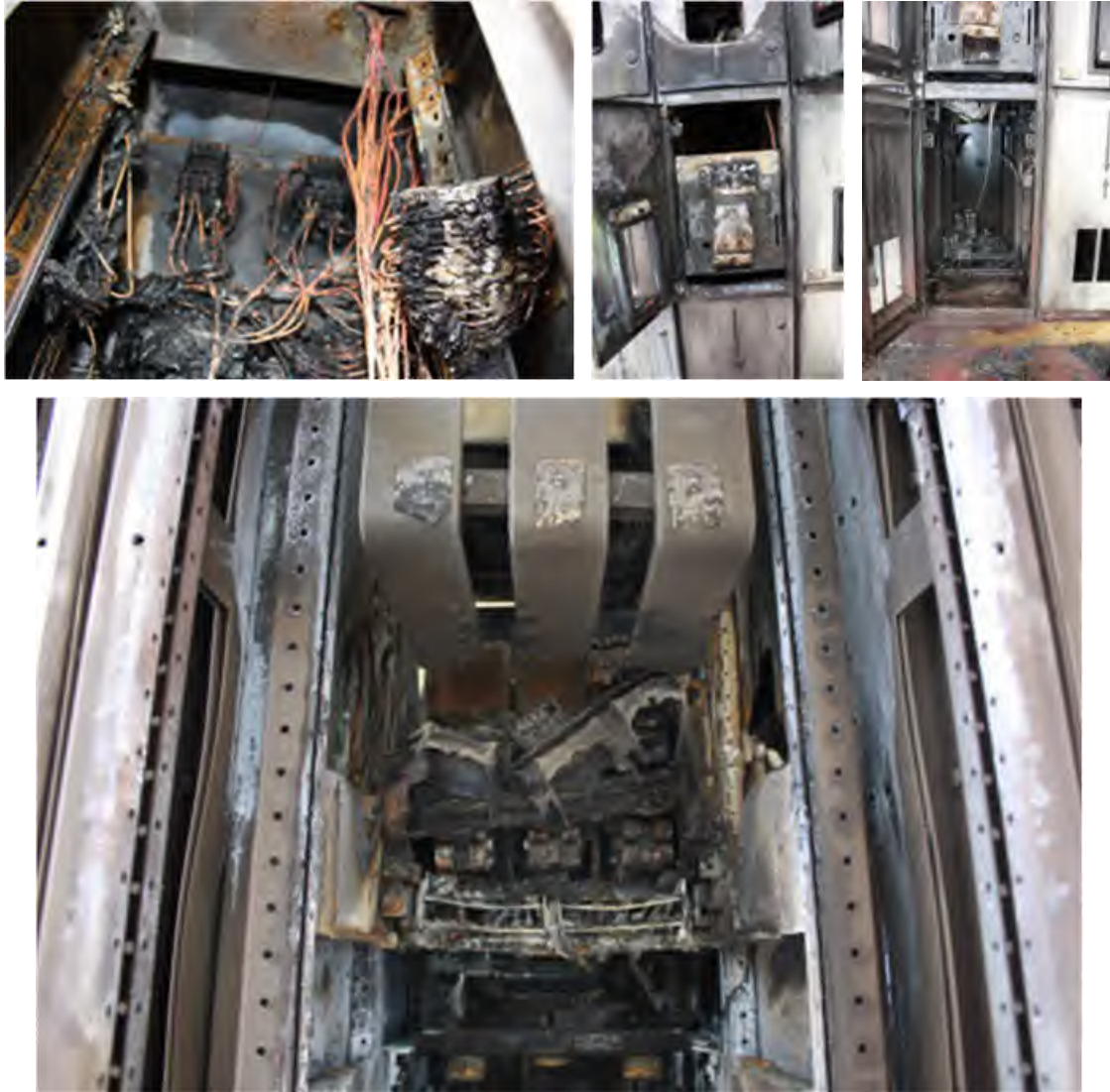
Fig. 170. Post-Experiment 2-33B Enclosure 'B' (EV52). Top left – upper cubicle internals showing remanence of panel wiring, Top center – middle cubicle with door open showing face of breaker, Top right – lower cubicle showing lower bus bars (all three phases) laying on floor of enclosure, Bottom – view of breaker from rear (note lower breaker stabs showing and lower bus bars are missing).
