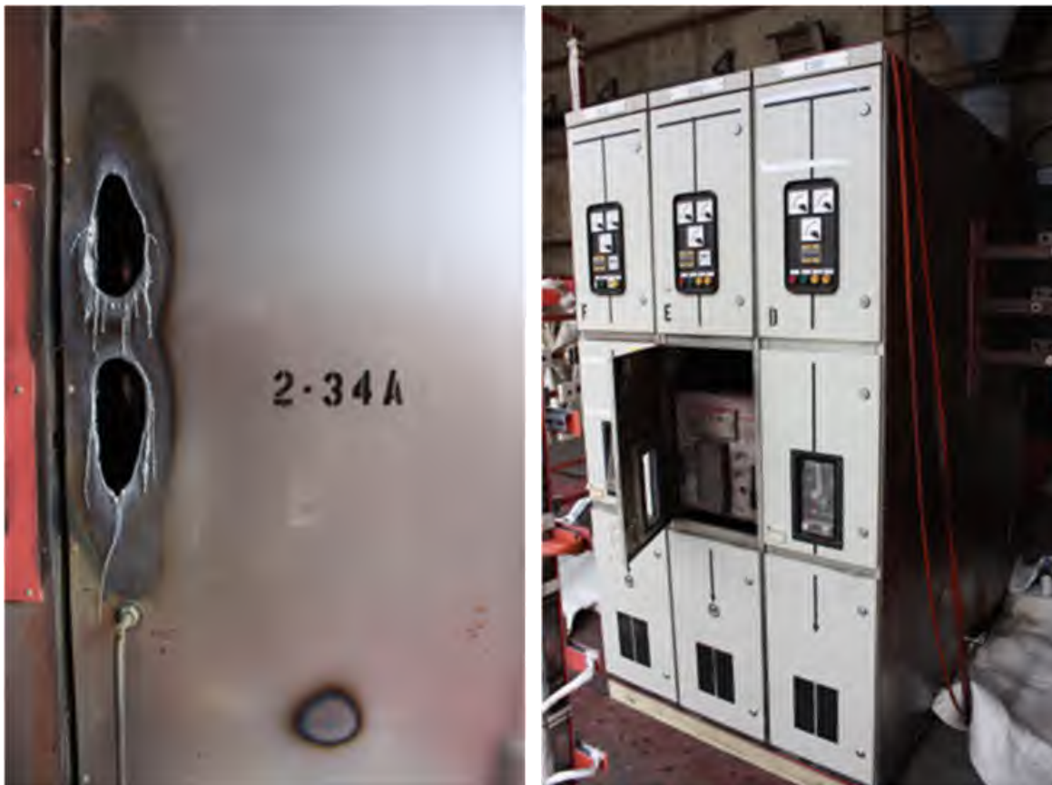
Fig. 43. Enclosures Post-Experiment 2-34. Left – enclosure breach on side of Enclosure ‘F’ (EU53), Right – front view of enclosures showing open door on breaker cubicle of Enclosure ‘E’ (EU52).
