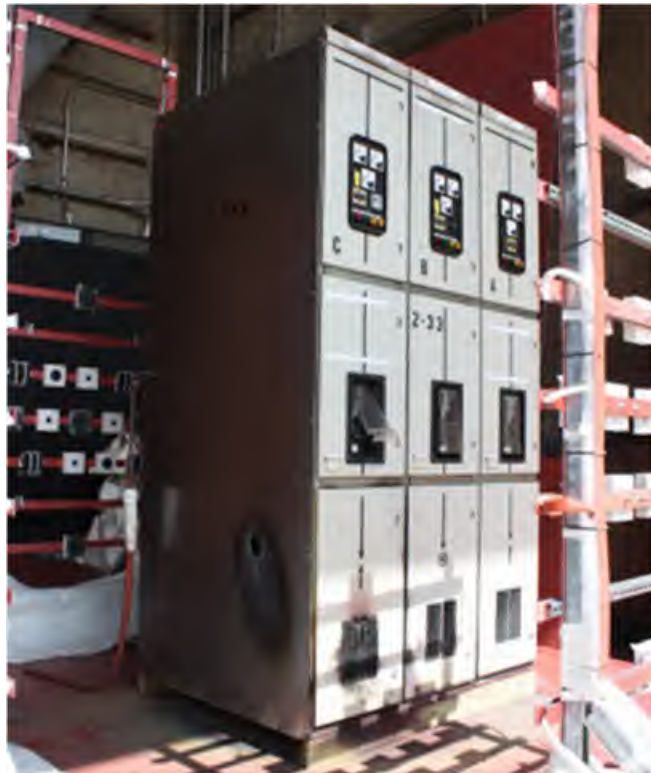
Fig. 162. Post-Experiment 2-33A. Note arc burn-through on side of Enclosure "C" (EV53), melting of vents in lower section and placement of breaker protection cover.
