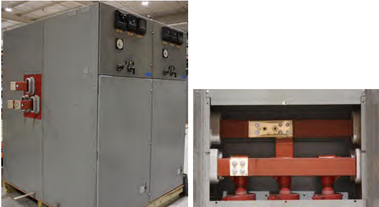
Fig. 186. Pre-Experiment 2-37 Enclosures “J” and “I”. Left – off angle view of Enclosure “J” (left) and “I” (right), Right – arc location main bus.
