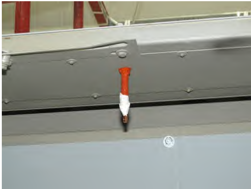
Fig. 22. Typical fiber optic sensor in top compartment of electrical switchgear, protected by silicone tubing and glass tape.
