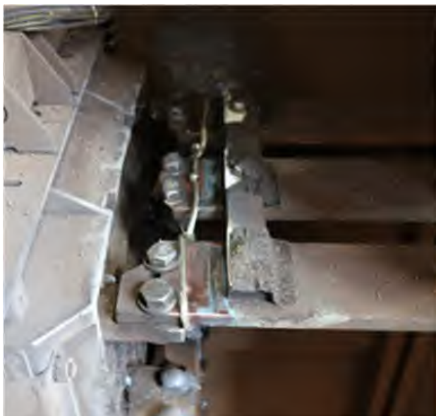
Fig. 222. Pre-Experiment 2-YYA. Arcing wire location.
