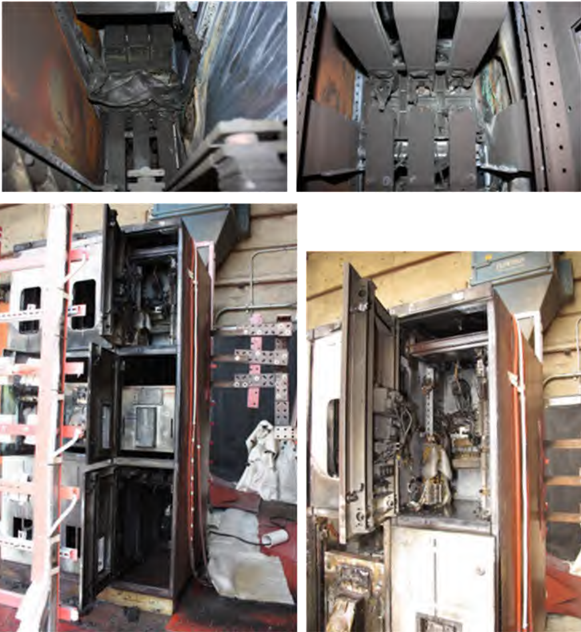
Fig. 169. Post-Experiment 2-33B Enclosure 'A' (EV51). Top left – top of breaker viewed from rear of enclosure, Top right – back of breaker, Bottom-left – Front of enclosure with all three cubicle doors open, Bottom-right – top enclosure close-up view.
