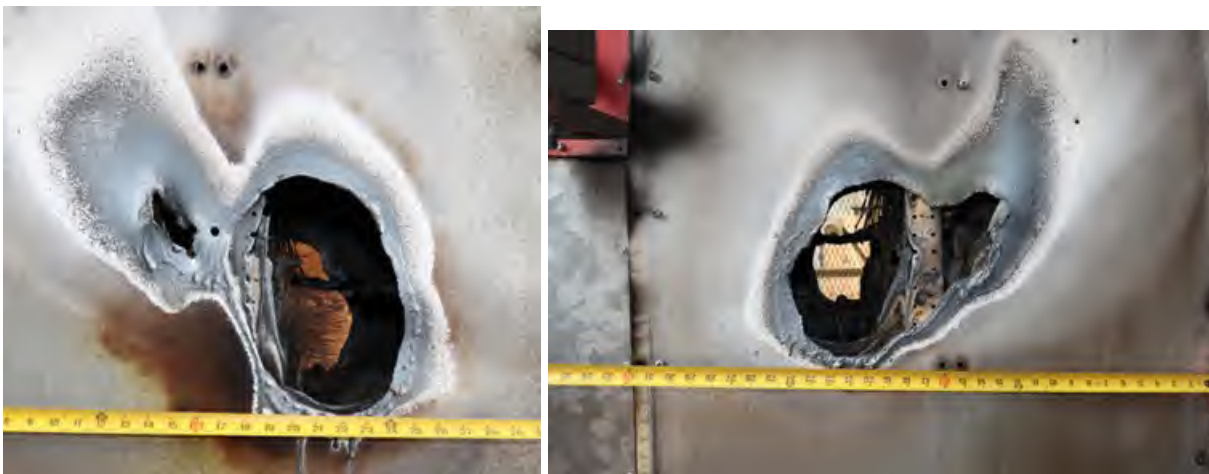
Fig. 224. Post-Experiment 2-YYB Enclosure Breaches. Left - enclosure breach on right side of enclosure (opposite incoming power supply), Right – enclosure breach on left side of enclosure (incoming power supply side). (cladding 1.5 mm [0.060 in] thick).
