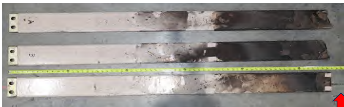
Fig. 82. Photo of Experiment 2-40 bus bars post-experiment (arc location at arrow).
