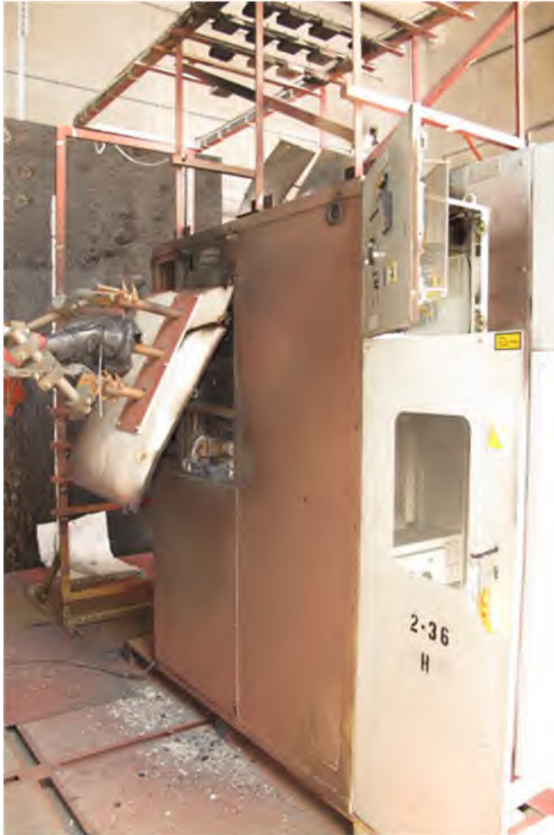
Fig. 55. Enclosure Post-Experiment 2-36. Note, the phenolic panel was separated from the switchgear side, and two adjacent top panels were deformed but remained attached.
