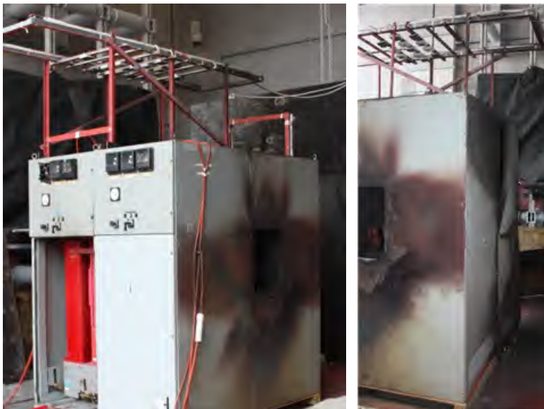
Fig. 63. Enclosure Post-Experiment 2-37. Door of Enclosure “J” was blown off, side panel of Enclosure “I” was blown off, and both rear panels were bowed.
